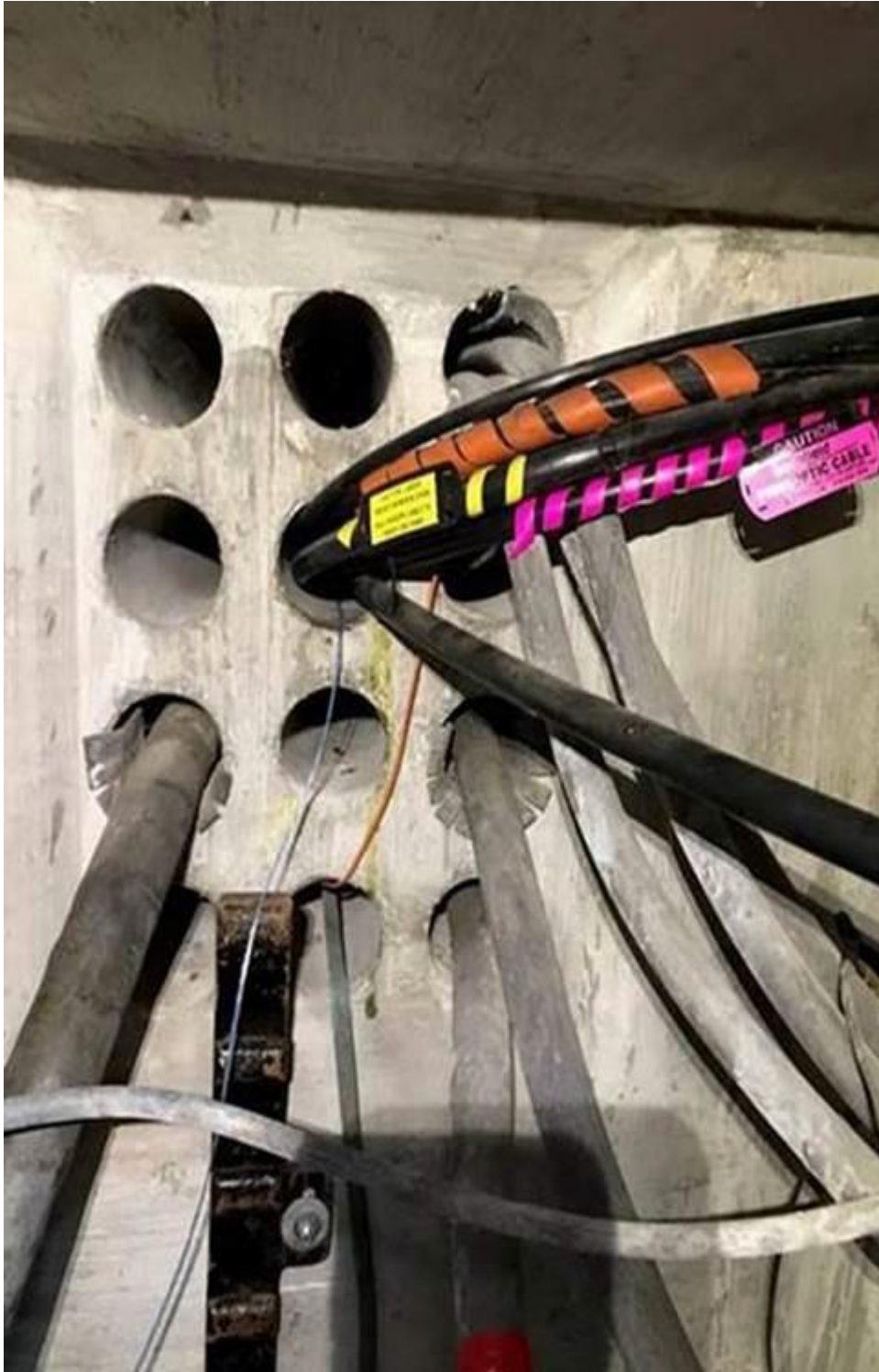
Typical Photo 3. Cable chamber with labelled cables
