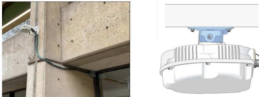
Fig 2. Images of an installed Aruba AP 565 with grounding
